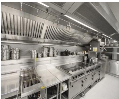
Exhaust Hood Ventilation for Cook Line Equipment
