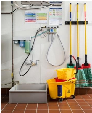
Janitorial Mop Sink
