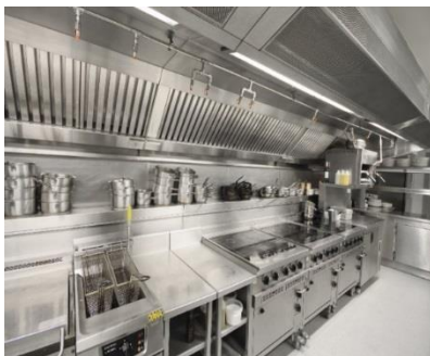
Exhaust Hood Ventilation for Cook Line Equipment
