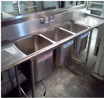
Three Compartment Sink
